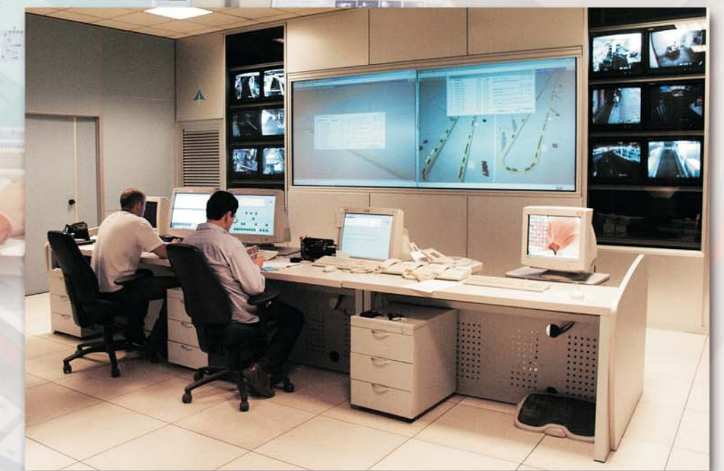
CENTRO DE CONTROL CONTROL ROOM
